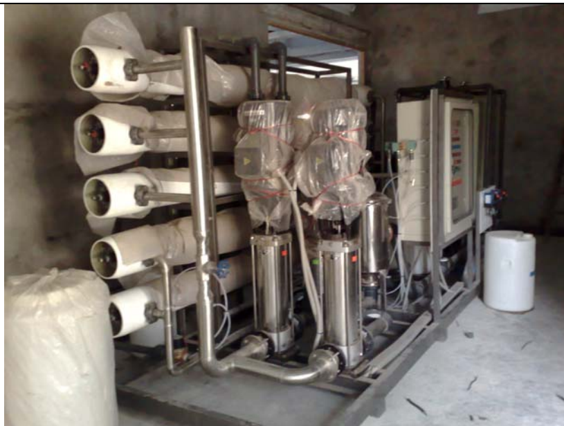
Reverse Osmosis plant: cap. 13.0 M 3 /hr.
