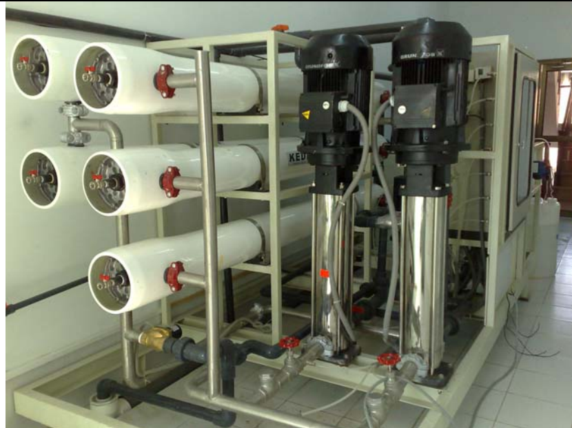
Reverse Osmosis plant: cap. 8.0 M 3 /hr.
