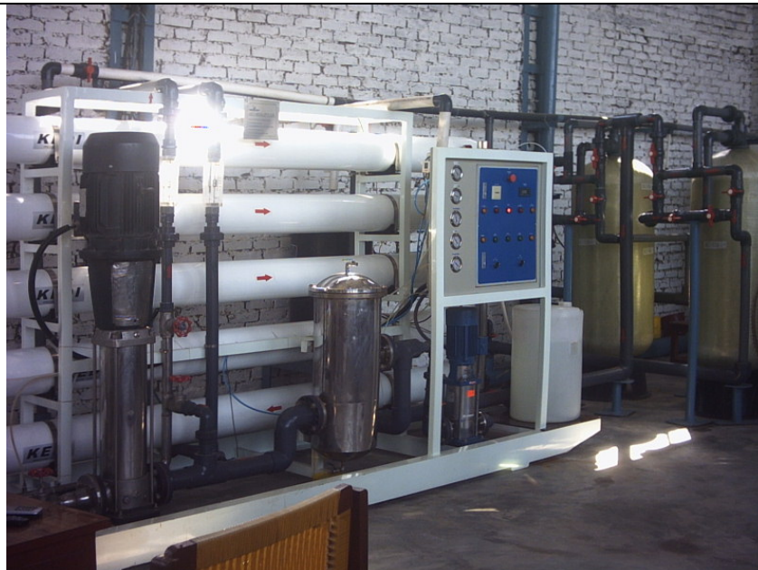
Reverse Osmosis plant: cap. 15.0 M 3 /hr.
