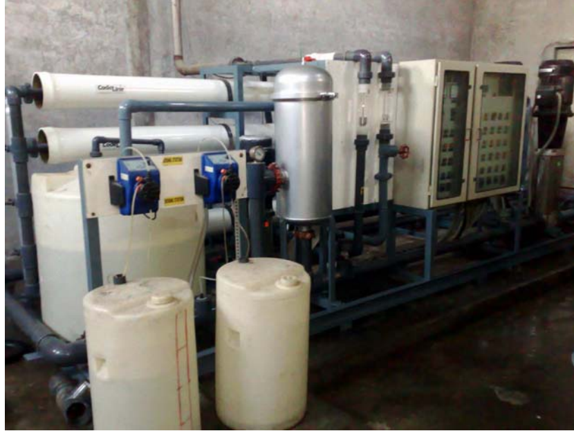
Reverse Osmosis plant: cap. 20.0 M 3 /hr.
